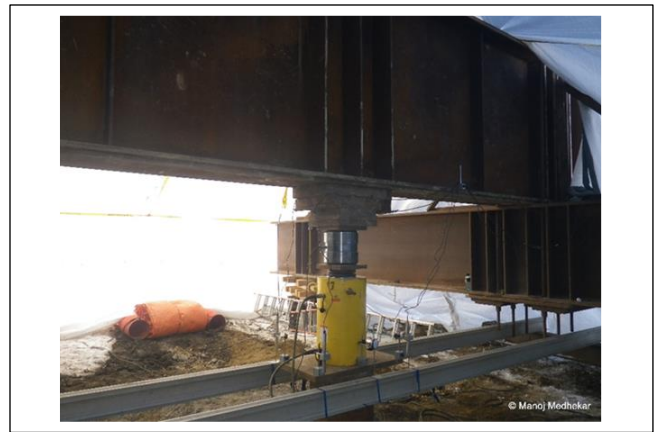
Fig. 3 - Static axial compression pile load test set-up at the Stony Plain Central High School.
