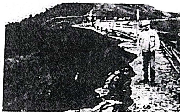
Fig.7 Failure of slope
